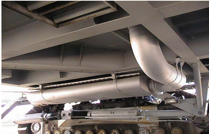
Figure 1: Old ALCO Engine Muffler and portion of old exhaust floor gratings
