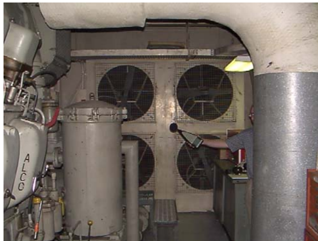
Figure 4: SPL Measurement in front of an Old Inlet Fan Set
