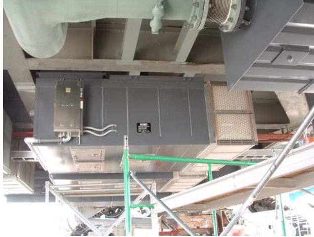
Figure 5: One of the 12 Acoustical Inlet Hoods under the CT with filtered air inlets
