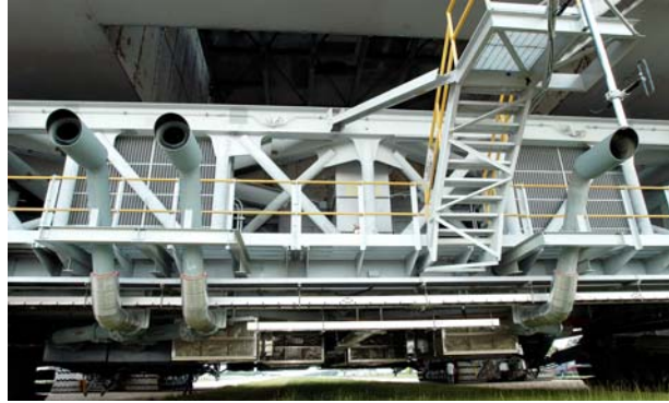
Figure 3: Extended Engine Exhaust Outlets terminating in front of radiator fans
